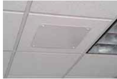
Installed Condition: PSIBVHF and PSIBVU78
